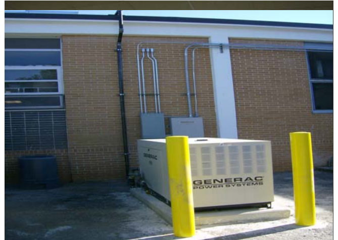
Shamrock MS New Generator and gas piping
