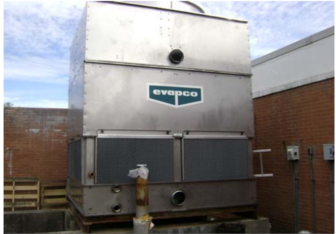
Sequoyah MS New Cooling Tower
