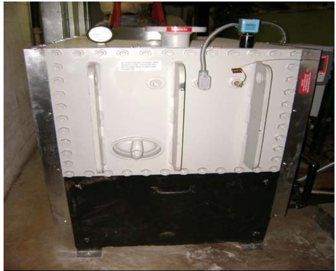
Sequoyah MS New Boiler
