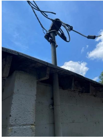
Power Pole Connected to the building
