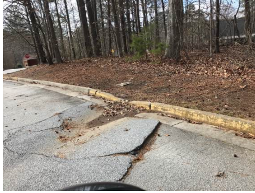
Fix Asphalt Damage
