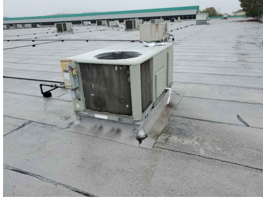
ERTU 22, 5 Ton Unit Shows Corrosion On Coil And Base. Replace These Units Have R-22 Refrigerant
