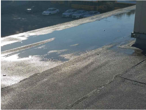
Puddling On The Roof
