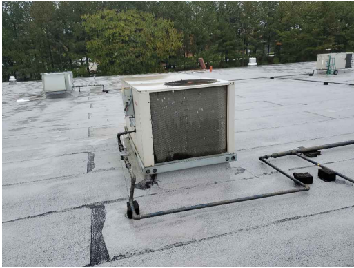
ERTU 20 Unit Coil Shows Corrosion And It Looks Like The Original Unit 5 Ton Unit With Gas Heat
