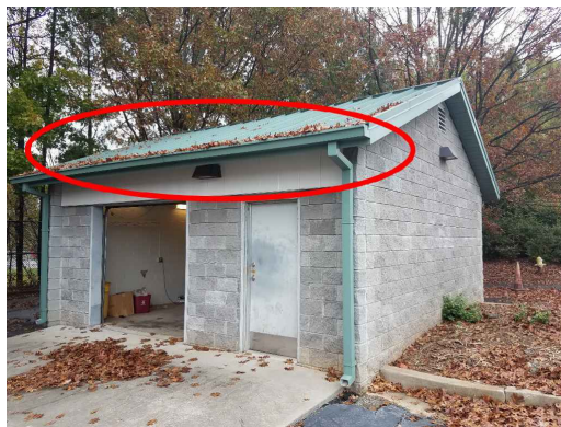
Gutter Needs Cleaning Of Tree Debris
