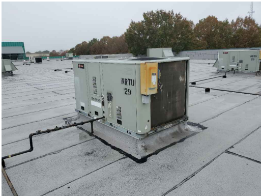
NRTU 29 , 10 Ton Unit Coil, Curb And Disconnect Showing Advance Corrosion. Replace
