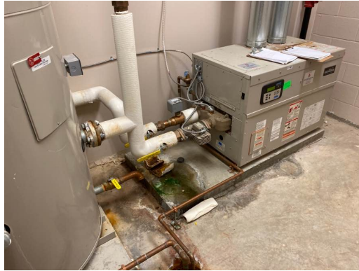
Gas Water Heater Is In Need Of Repair. Water Is Leaking Around Gaskets And Relief Valve
