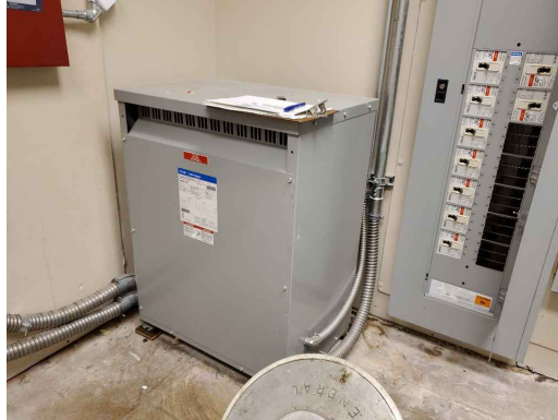
75KVA XFMR For Ldb
