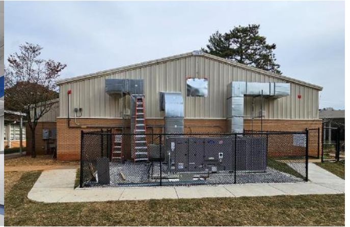
New HVAC Equipment
