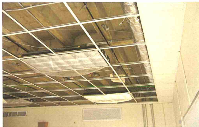
Avondale HS Ceiling Grid & Air Duct
