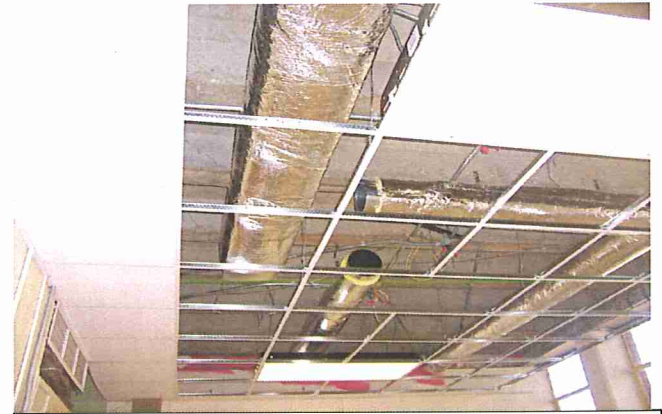
Avondale HS Supply Ducts
