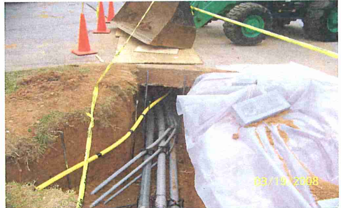
Jolly ES New Electrical Service
