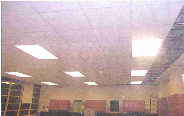
Avondale HS Ceiling Grid & Lighting
